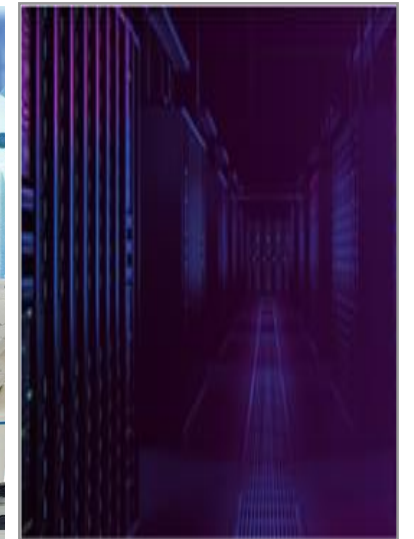
Data Center Precision Air-conditioning
